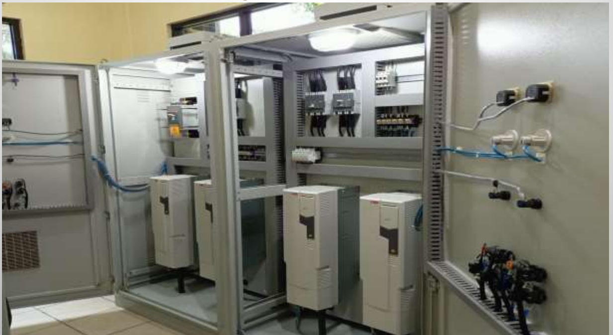
Panel VSD Aerator 4 x 55kW - WWTP Customer : PT. Kawasan Industri Mitra Karawang Location : Karawang Barat
