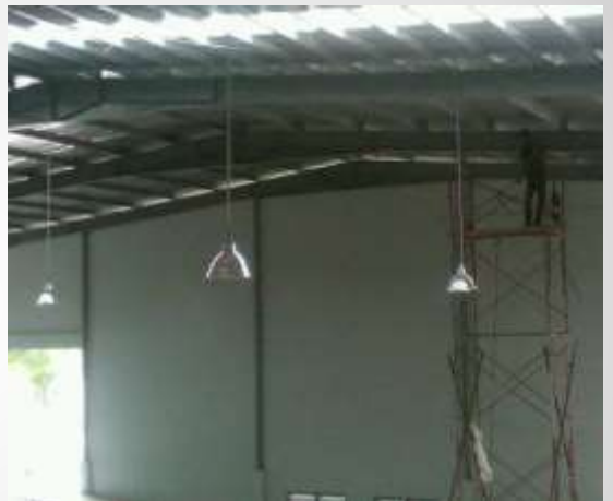
Product Name : Inst.Cable & Lighting Customer : PT.Cerestar Flour Mills Location : Cilegon - Banten
