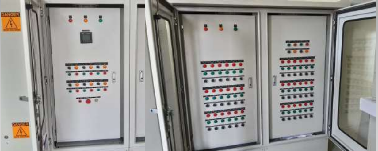
Panel MCC-1-2, Chemical dan Mixer, SCADA
