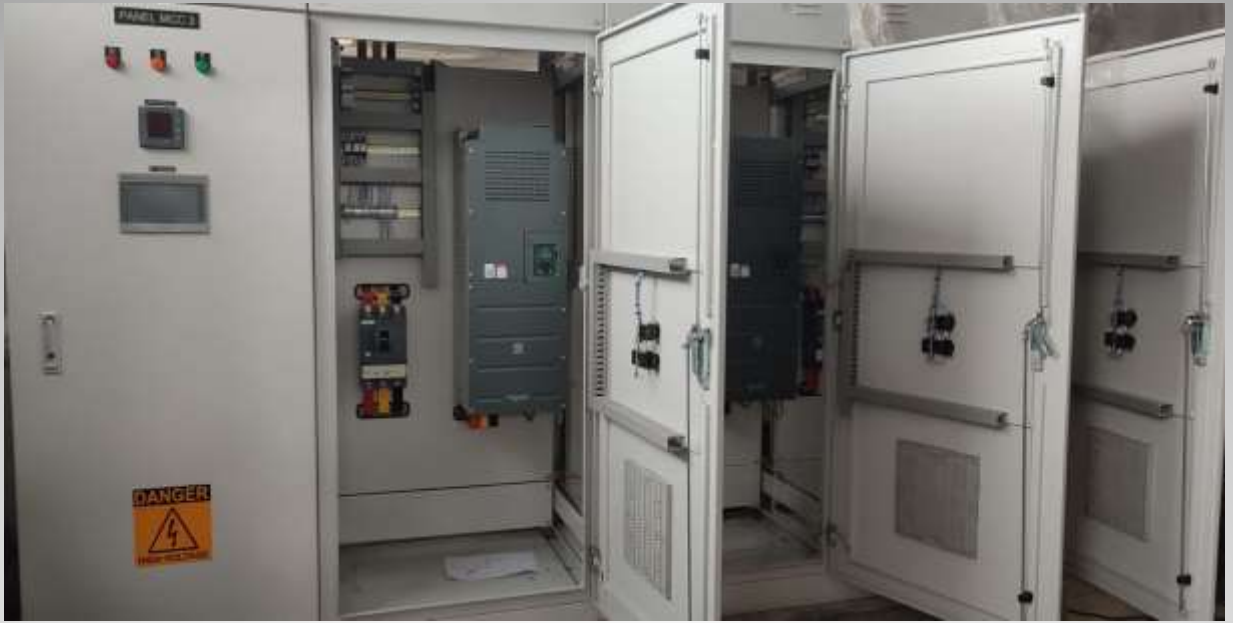
Panel MCC-3, Kabel Power Pompa Customer : PT. GRAHA CIPTAYASHA Location : Deltamas Cikarang
