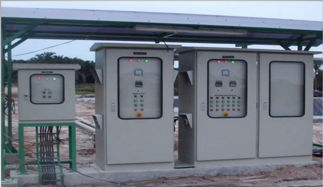
Product Name : Central Distribution Board Customer : PT. Nusantara Water Centre Location : Bangka - Belitung
