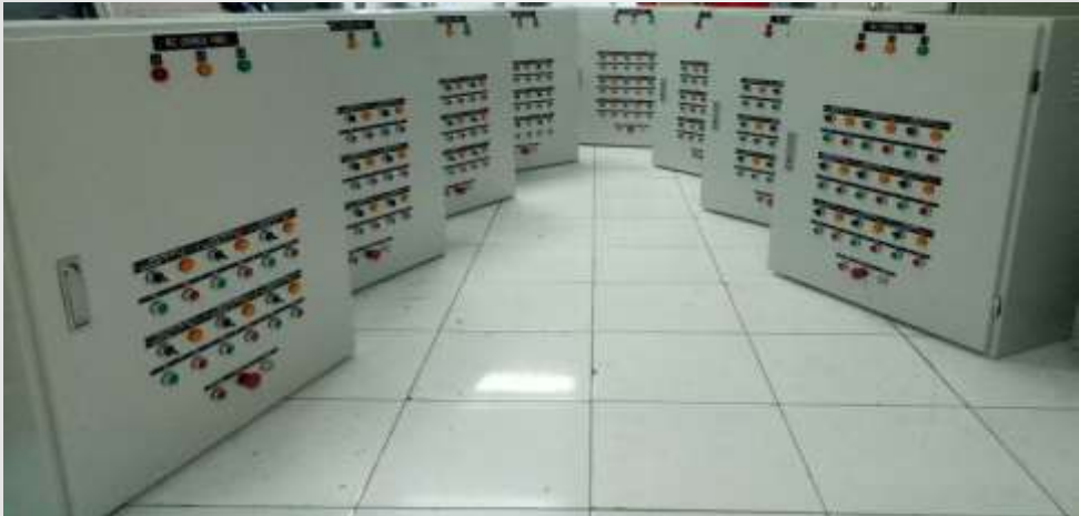
Panel Dosing System Customer : PT. Artha Envirotama
