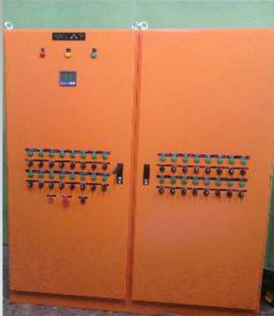
Product Name : WWTP Panel Customer : PT. TirtaKreasi Armita Location : Bentoel- Jakarta
